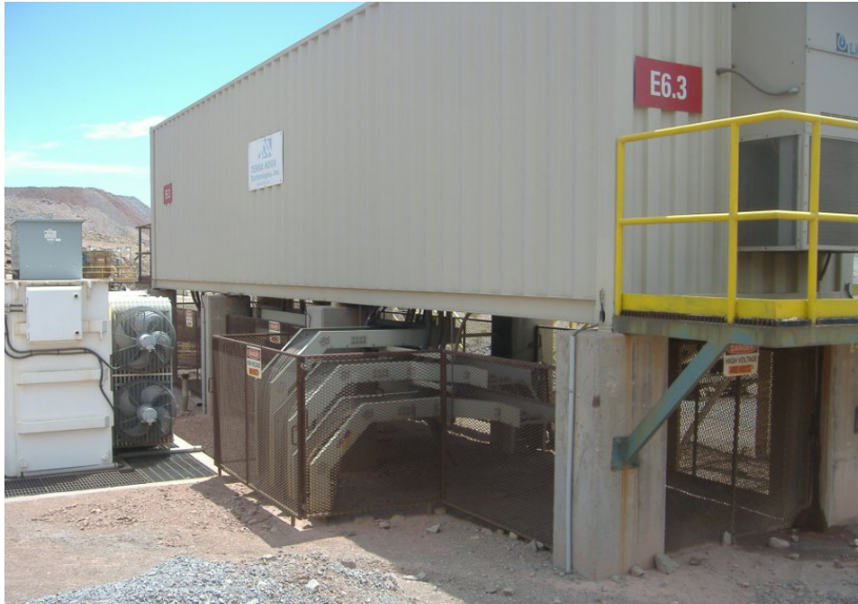
Figure 10: Prefabricated electrical room
