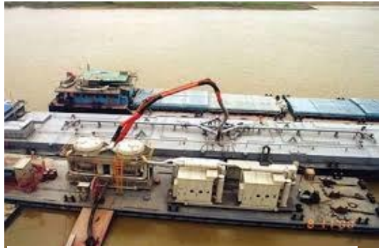
Figure 8: Barge Mounted Unloader (Photo courtesy of FLSmidth)
