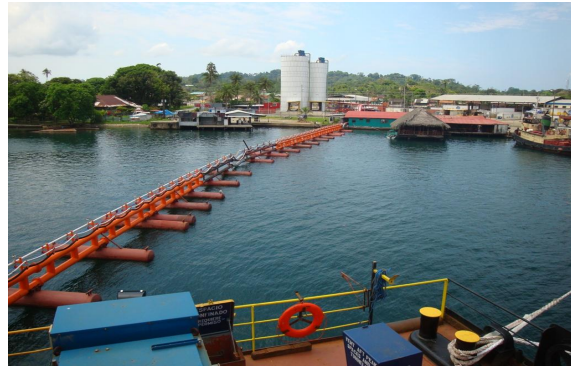
Figure 7: Floating Pipeline to Truck Loading Bins
